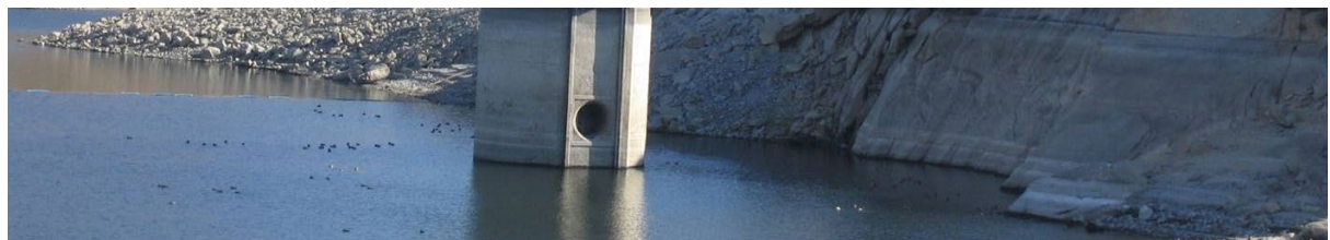
Seismic retrofit of the Perris Dam. Photo credit: California Department of Water Resources, 2019.
