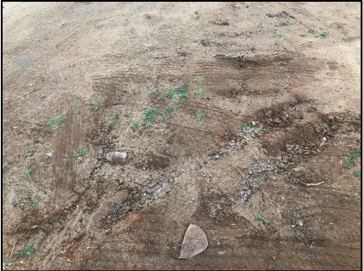
Figure 4.1-6 NATIVE SOIL NOT COVERED WITH GRAVEL
