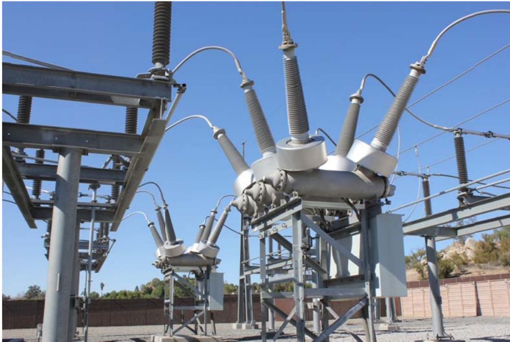
115 kV Circuit breaker
