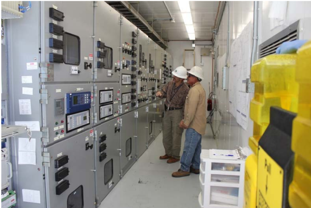
Inside Switchgear building
