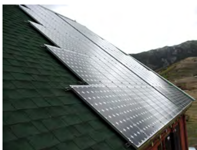
Monocrystalline solar panels.
