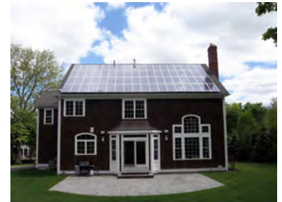
Roof-mounted solar array for large power capacity.
