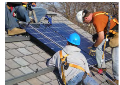
Crystalline solar modules mounted on aluminum racks, with airspace to keep them cooler.
